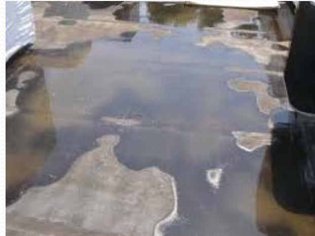
Clogged drains and ponding
