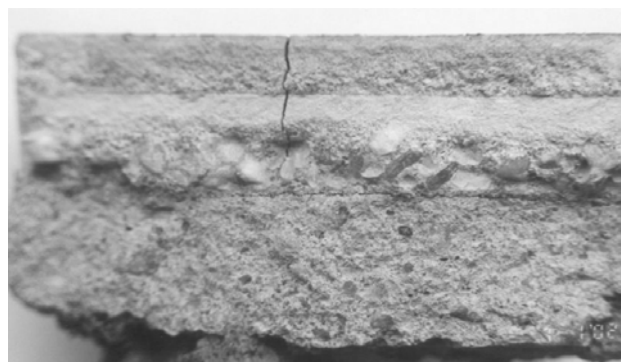
Figure 4 - Cracking and curling of leveling mortar (Beasley)
